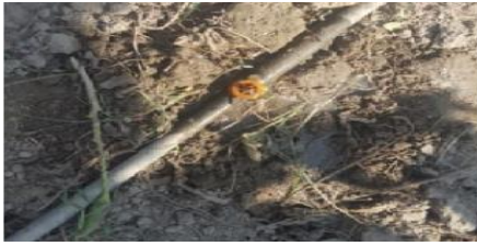
Fig.7 Dripper installed at the lateral piping
